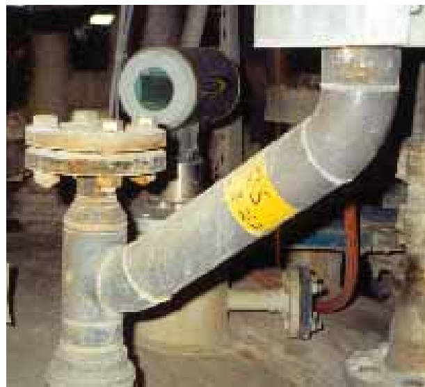
The Siemens radar instrument provides reliable level measurement even in the harsh conditions of this dioxide reactor tank, using a purging kit to periodically clean the antenna without interrupting the process.
