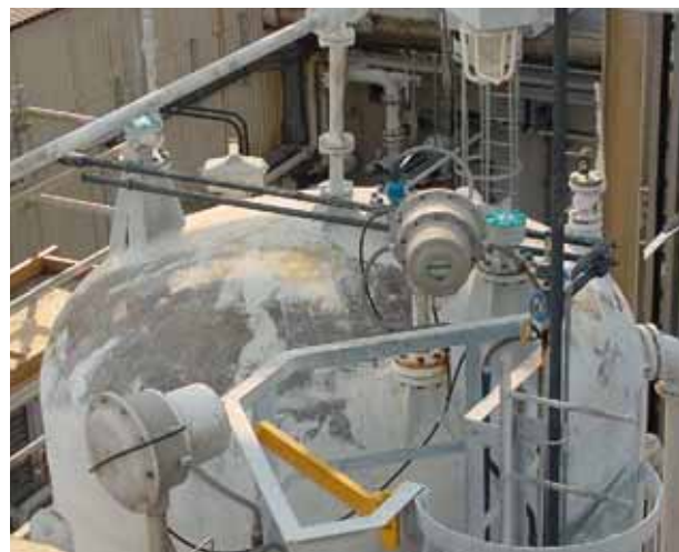
Reliable interface measurement helps Dow maximize productivity in its agricultural products plant in Freeport, Texas.
