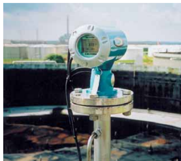
Installing waveguides with IQ Radar instruments solved a difficult measurement problem for BP Lubricants in Hamburg without the need for costly modifications to the existing tanks or flanges.
