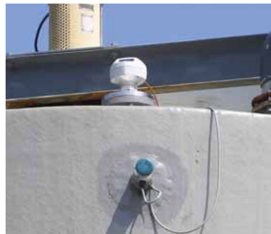
A Siemens SITRANS LR 200 radar transmitter mounted on the top of the tank provides continuous level measurement, while a Pointek CLS 100 capacitance switch provides a high level failsafe. Both instruments are installed outside the tank wall.
