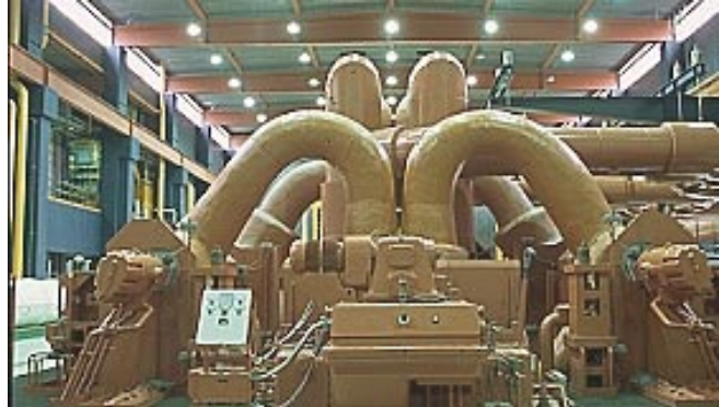
From the generator gallery in Block 5: turbine and generator
