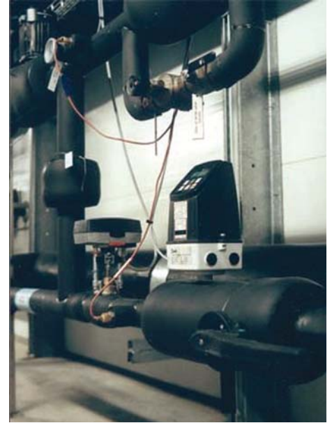
SITRANS F M electromagnetic flowmeter installed in the water supply.
