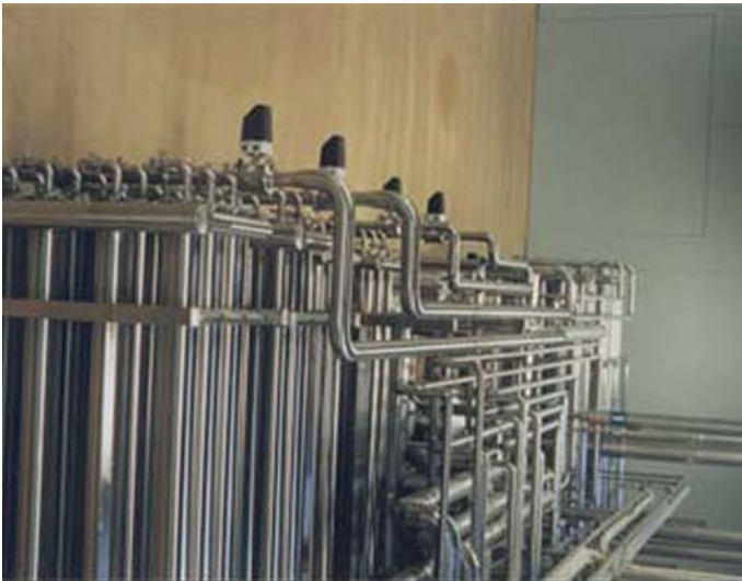
MAG 1100 FOOD flowmeters installed in the concentration plant for the curdling process.
