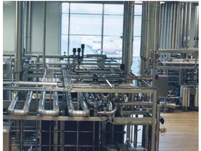
MAG 1100 FOOD flowmeters installed in the membrane filtration plant for whey processing.
