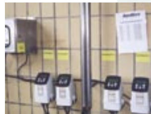
A close-up on the transmitter conveying data from the flow sensors. Two of them control the dosing of antioxidant, while the other two control the addition of foam stabilizer.
