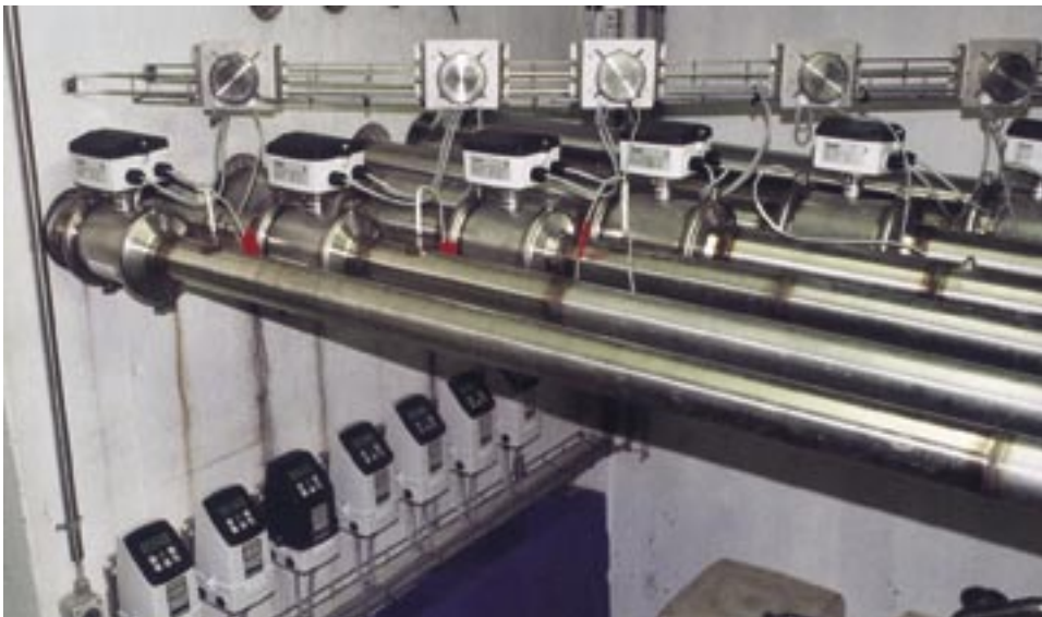
Flowmetering of the weighing procedure is managed by seven MAGFLO electromagnetic flowmeters. One of these meters was inaccurate because of cross-mounted cables.
