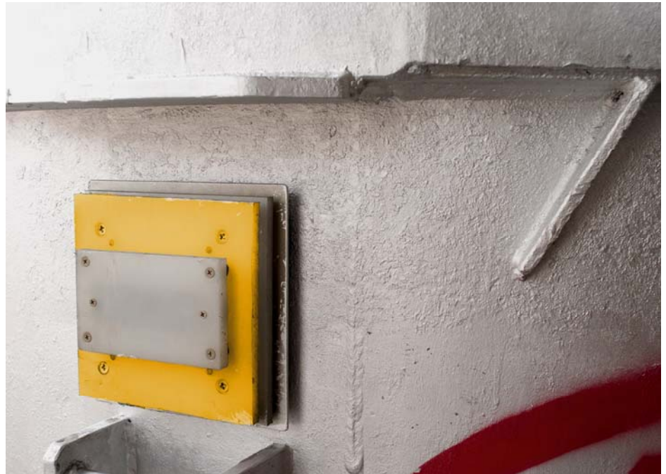
The high external temperatures are dissipated to the ambient air through a multilayered design so that the SIMATIC RF620T transponder (below the white cover plate) is operated within the specification.
