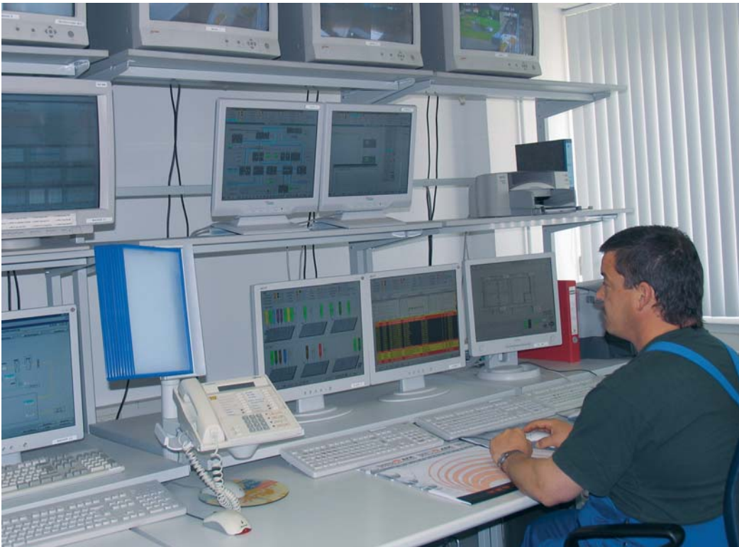
All of the information converges at the new PCS 7 control center
