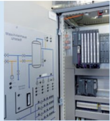
Each of the 11 local and 14 decentralized units is equipped with a Simatic controller and an operator interface
