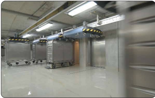
Figure 1: Particularly at mealtimes, there are busy scenes in front of the elevators in the main ward building. Everything is managed quickly, safely and without collision by the control network.
