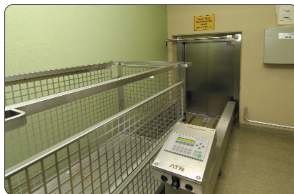
Figure 3: Combined PLC and operator panel
