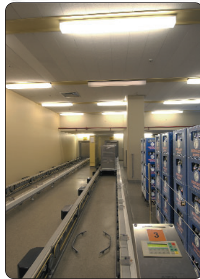
Figure 2: After entering the destination number on the Simatic OP3 operator panel, containers are automatically transported to the relevant floors from the dispatch store to the supply floor.
